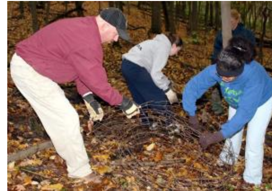
Greg Orr (Anderson) and Rocio Garay (Anderson) work together to remove old fencing at Anderson Park District's Johnson Hills Park for Make A Difference Day.
