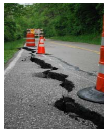
A landslide pulled apart a culvert pipe and cracked the pavement on Elstun Road.
