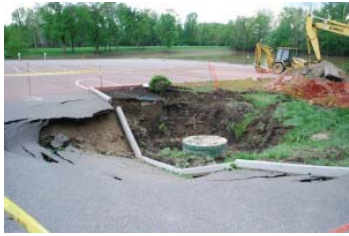
A sinkhole swallowed a manhole cover at the entrance to Kellogg Park.
